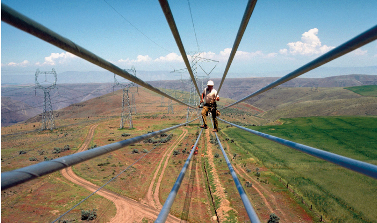
A worker inspects Bonneville Power Administration lines in Oregon in the 1970s. Credit: James L. Amos via Image Bank Unreleased/Getty Images.
