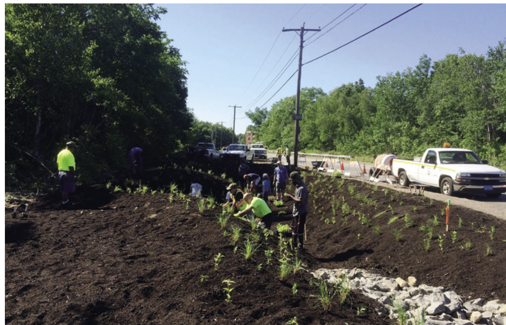
Volunteers helped the Worcester Department of Public Works and Parks install a rain garden along a busy road in the northeast section of the city. Credit: Worcester DPW
