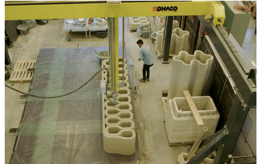
Construction of the printed houses will be similar to the bridge-printing process shown here, with various elements built in the university's lab, then transported and assembled at the site of the planned development. Credit: Imagecollectors.
