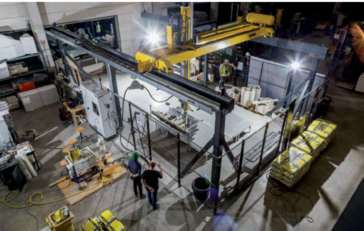
The large-scale 3D technology that will be used to print the houses, shown here, was pioneered at the University of Eindhoven and used to build the world's first concrete 3D-printed bridge. Credit: Imagecollectors.
